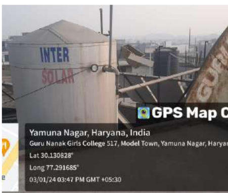
Solar Water heater
